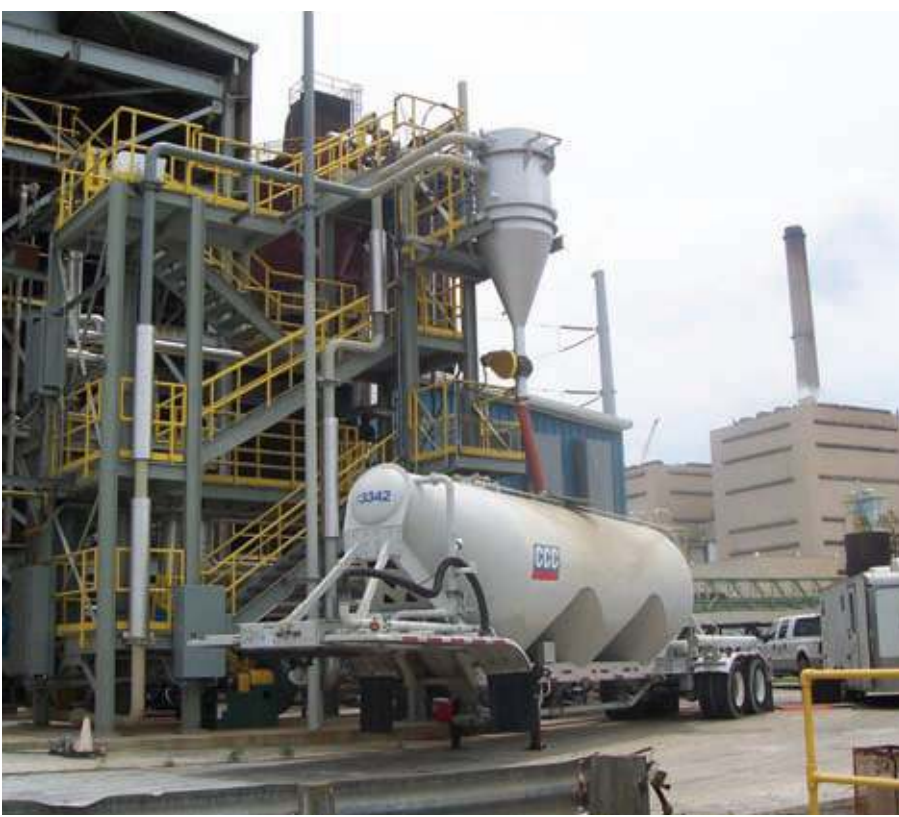
Figure 2. PMI Ammonia Recovery/Removal Pilot Plant.
